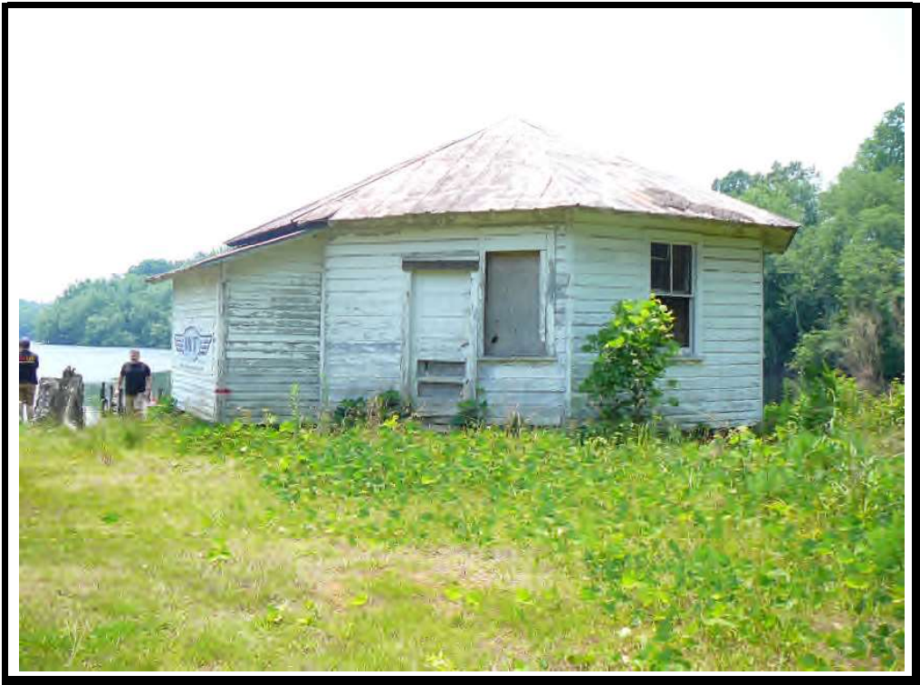
#2 - View South of the Old Boat House (To Be Razed) on the Subject Property Taken By Cedar Creek Appraisals 6/8/2023
